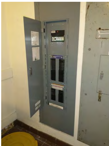
Photograph 1: View of electric panel in room no. 5C32.
