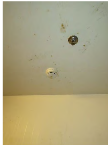
Photograph 2: View of smoke alarm in room no. 5C32.
