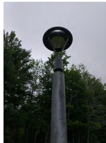
Photograph 4: View of LED exterior Lights.
