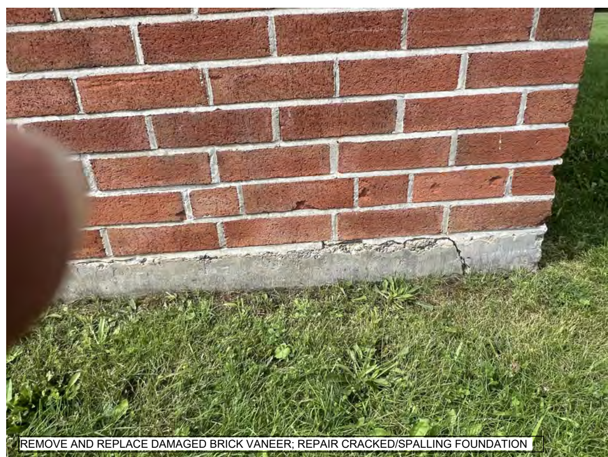
REMOVE AND REPLACE DAMAGED BRICK VANEER; REPAIR CRACKED/SPALLING FOUNDATION
