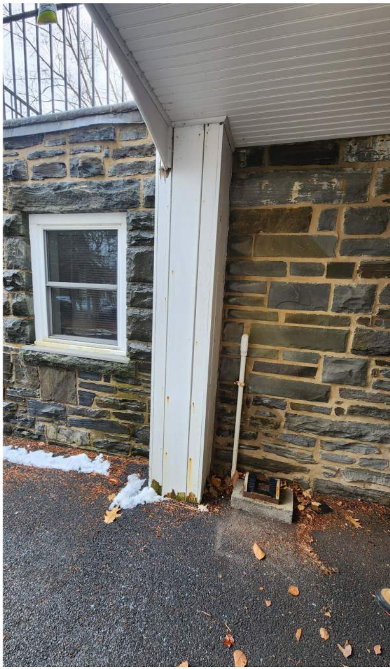
Exterior view of north basement wall. Secondary service entrance enters basement electrical closet approximately 18"-24" west (right) of window pictured. Remove and replace framing in-kind to replace secondary electrical service.
