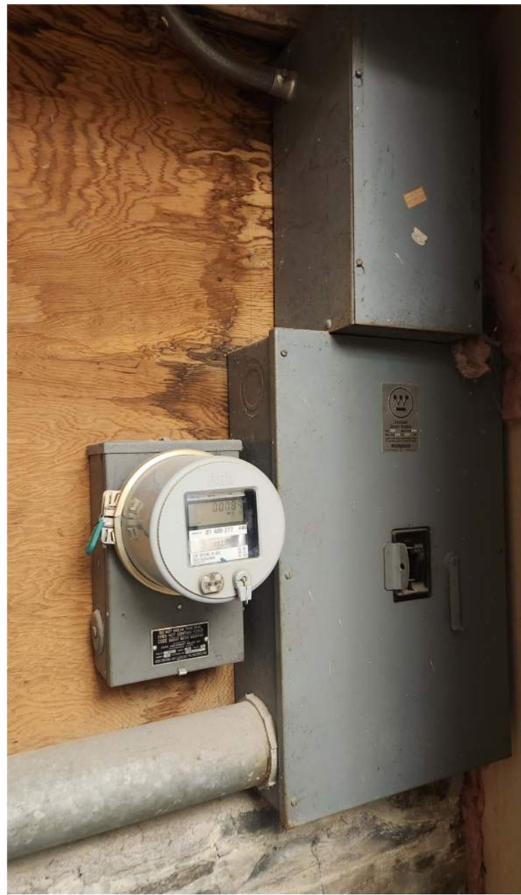
Interior view north basement wall. Due to electric panel and meter locations, it is assumed that secondary service enters the basement above finish grade. Contractor must provide all materials and labor to replace secondary service and repair building and framing in-kind.
